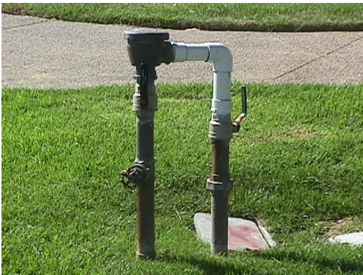
Figure 3. Pressure Vacuum Breaker (PVB).
